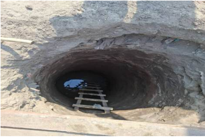
Figure 2 : excavation of the selected sites
